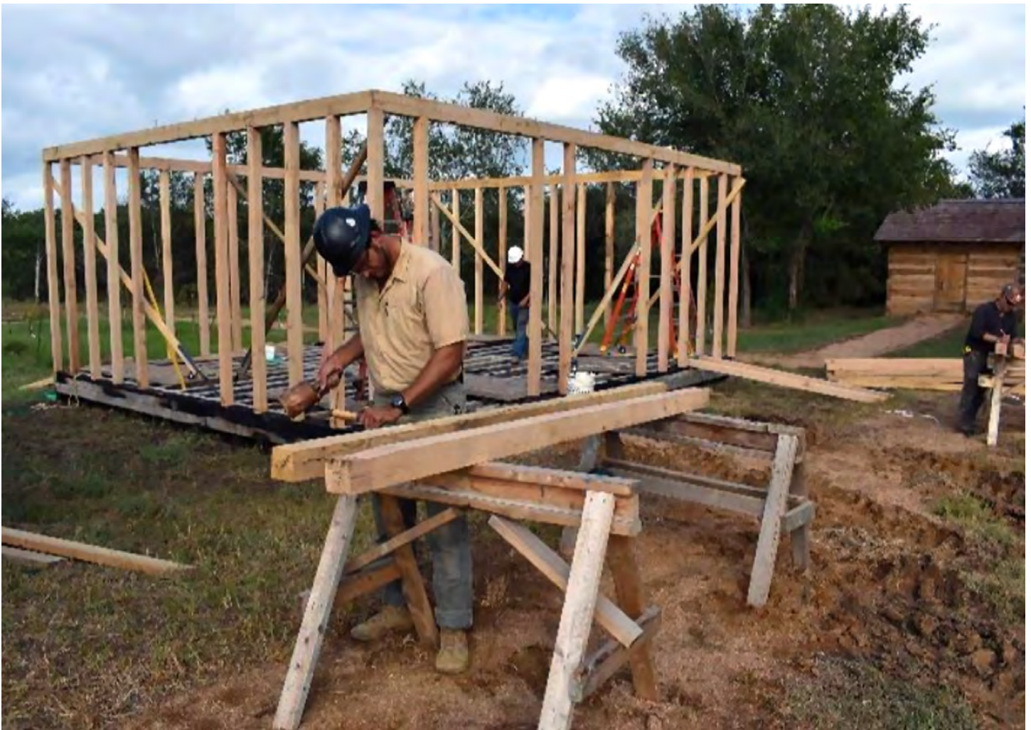
Assembling the reconstructed Courthouse's timber frame, September 2021. Photo courtesy of the Texas Historical Commission.
